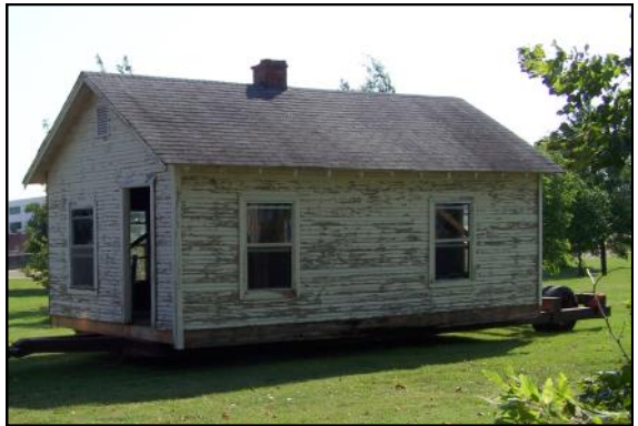
The exterior of the building will require paint, new windows, a porch and steps.
